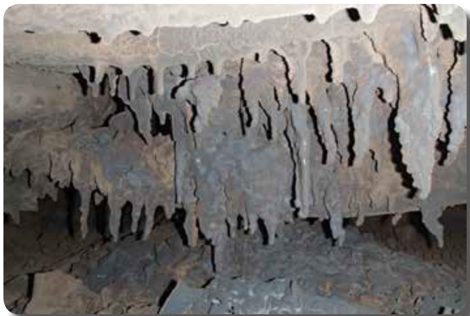
Fire damage to EGE
